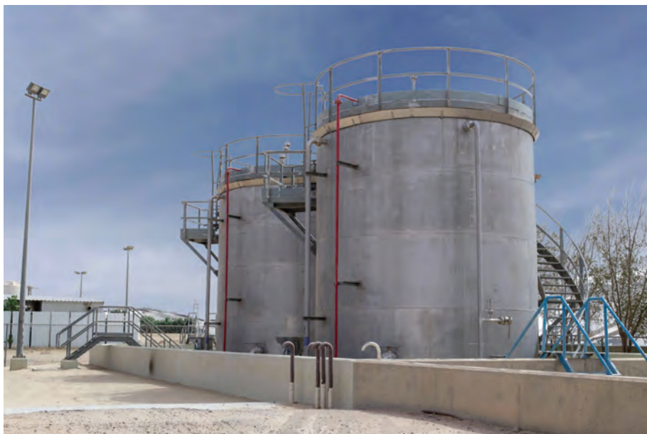
New tanks and associated piping at the Wafra Oilfield's bulk chemical handling facility were constructed with Type 316 and Type 316L SS.
