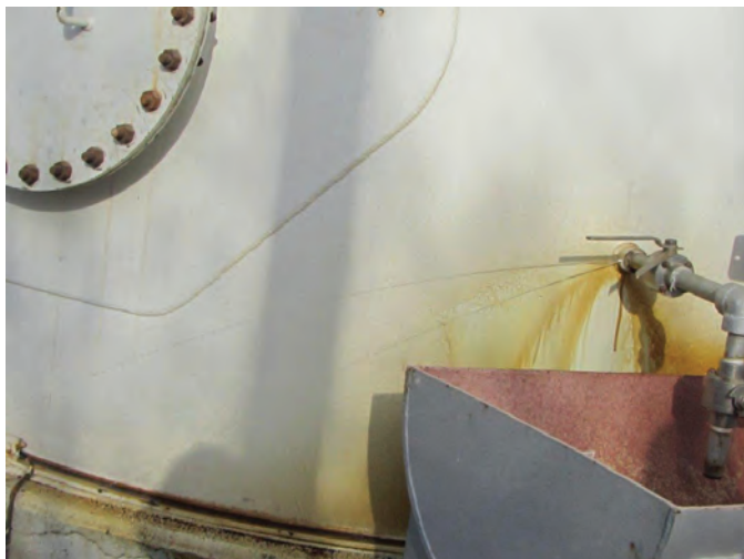
Chemical leaked at the welding joint on the tank sampling point.
