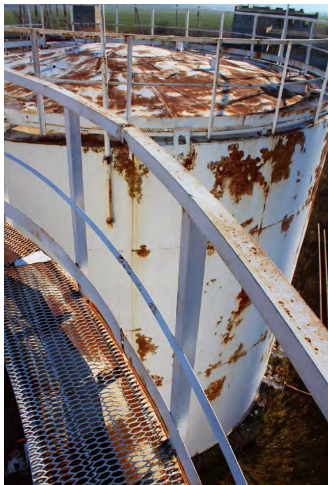
Corrosion is a leading cause of storage tank failure. Fortunately, there are many ways to prevent this problem.
