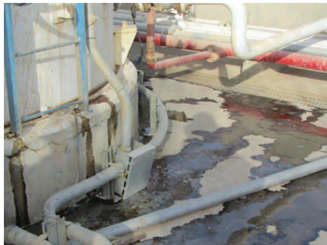
Chemical spillage around the periphery of the tank.
